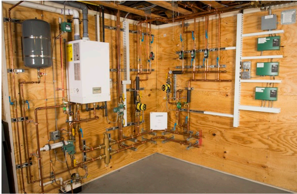
The mechanical room.
