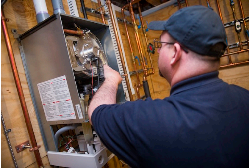
Golden checks the Viessmann Vitodens 100 condensing gas boiler.
