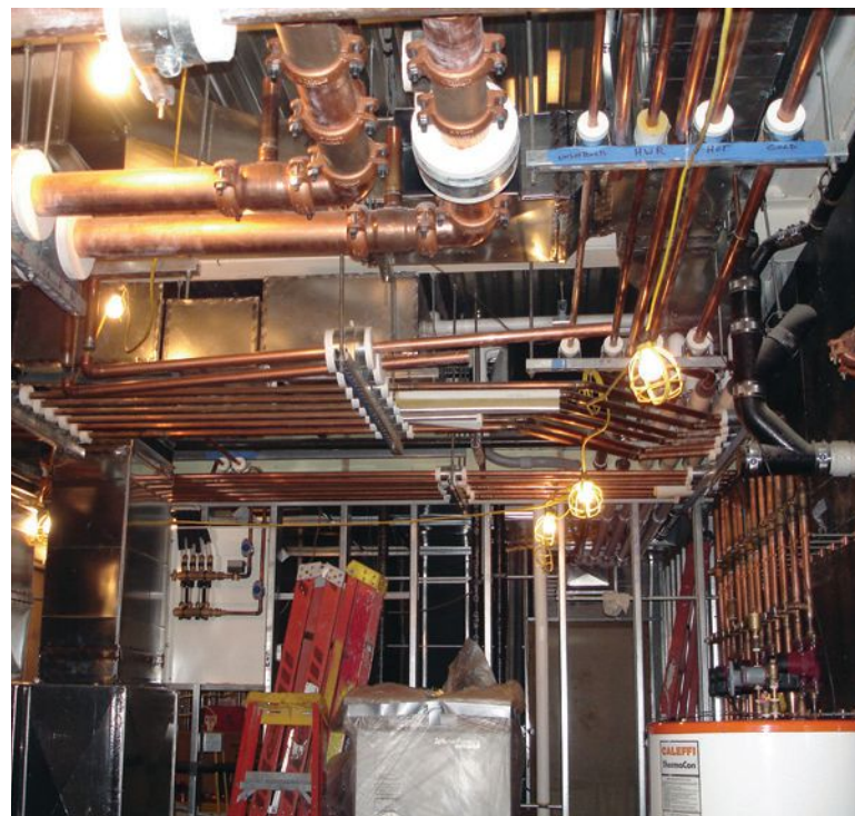
Ceilings often get crowded once piping for geothermal, radiant, air distribution, and plumbing systems are installed. (Courtesy of William Jannone & Sons Inc.)
