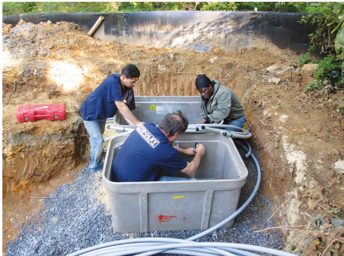
For this private residence in Bethesda, Maryland, Foley Mechanical technicians install geothermal manifolds in a concrete vault.
