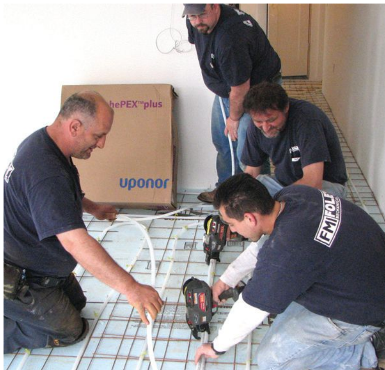
Technicians from Foley Mechanical install 1/2-inch PEX-a tubing in an application in Washington, District of Columbia.
