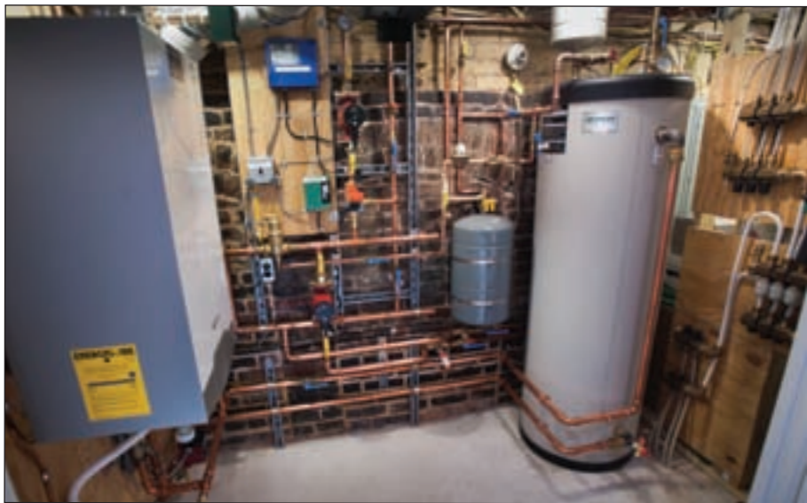
Foley Mechanical technician Brian Golden did a masterful job fitting the Triangle Tube boiler and tank, Uponor manifolds and boiler piping in this tight mechanical closet.
