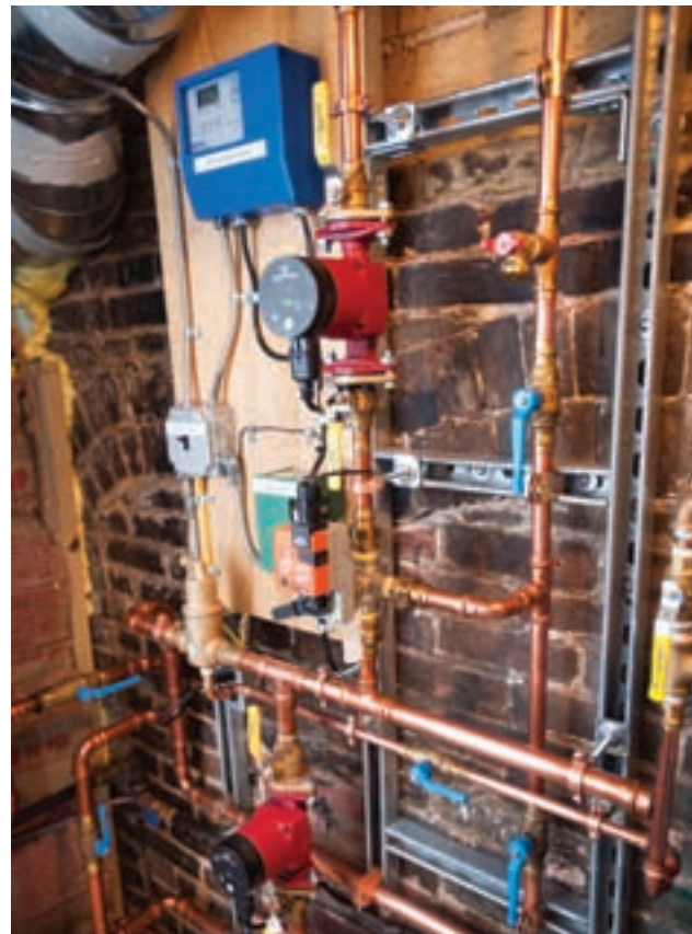
Grundfos variable speed pumps provide flow for the radiant zones and DHW tank. Cimberio press ball valves provide isolation for the hydronic components.
