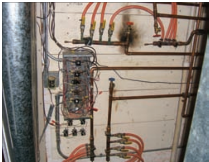
At the manifolds, several of the barbed fittings were leaking. The tubing was becoming hard and brittle.
