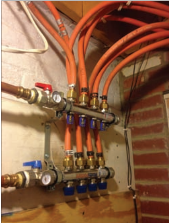
All the manifolds were replaced with new stainless steel manifolds with integral balance and isolation valves.
