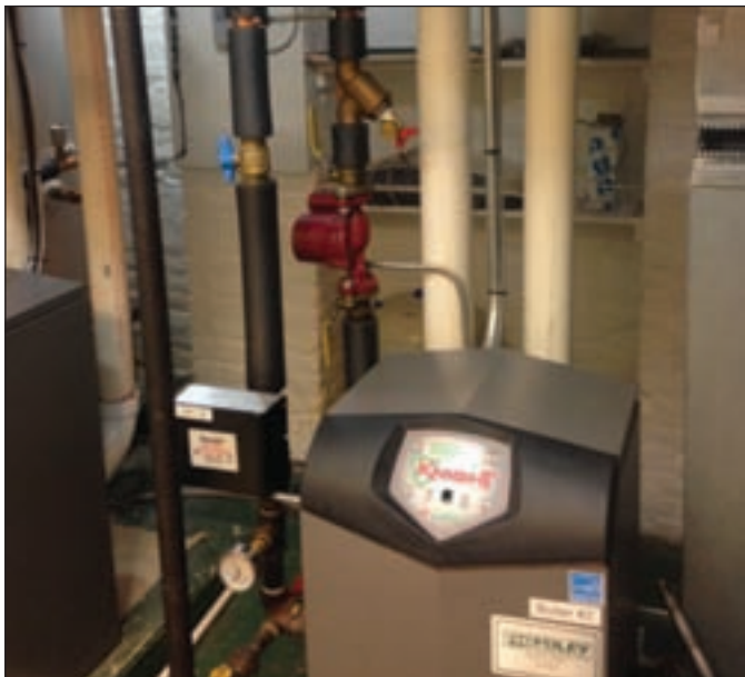
After the system was clear, refilled and purged, we introduced two gallons of boiler treatment.
