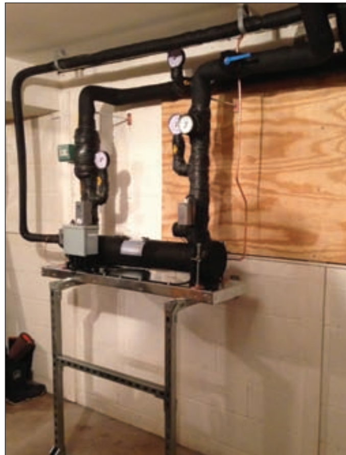
Photo 3: Reverse angle on the standard chiller barrel heat exchanger.
