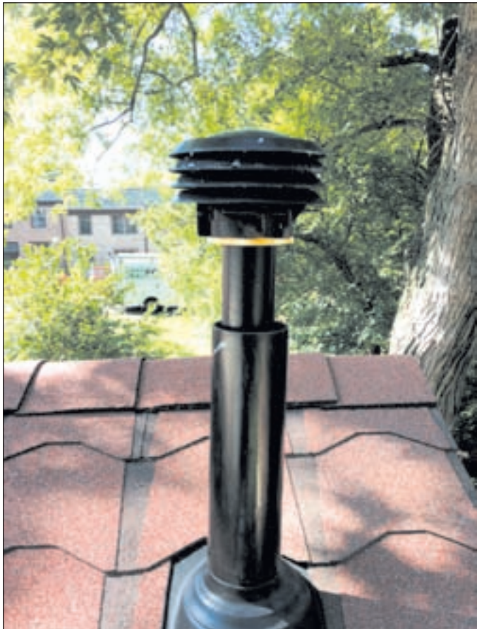
Photo #1: The vent cap on the boiler concentric vent kit was replaced by the roofer with a PVC bushing and B-Vent termination without informing anyone.
