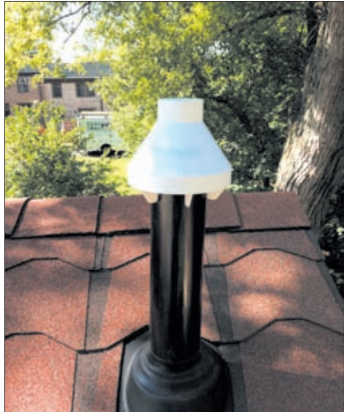
Photo #2: Boiler concentric vent kit with the correct termination installed.
