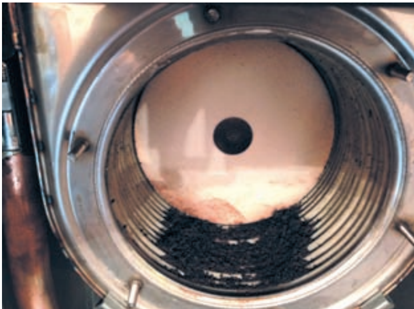
Photo #3: Debris in boiler heat exchanger caused by incomplete combustion due to recirculated flue gases.
