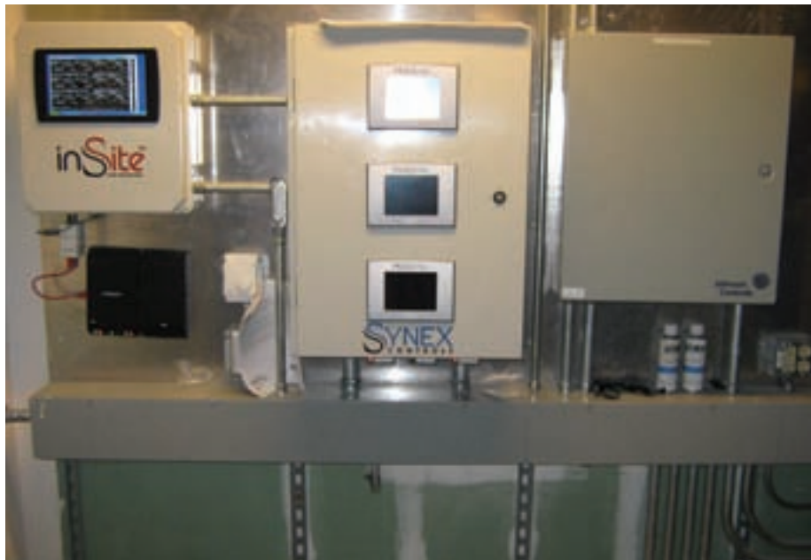
The bank of Fulton boilers is controlled through a custom DDC control system that allows David LeMay as well as Lambeau staff to monitor and control the system remotely.
