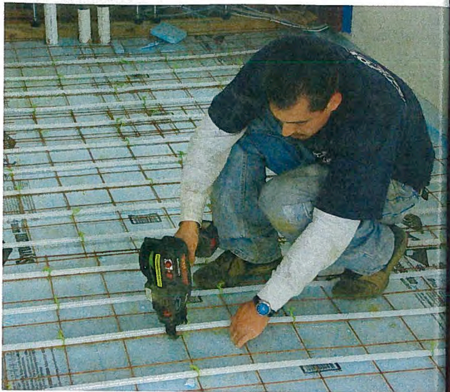
Foley Mechanical had two days with a 12-man crew to lay 15,000 feet of PEX tubing.
