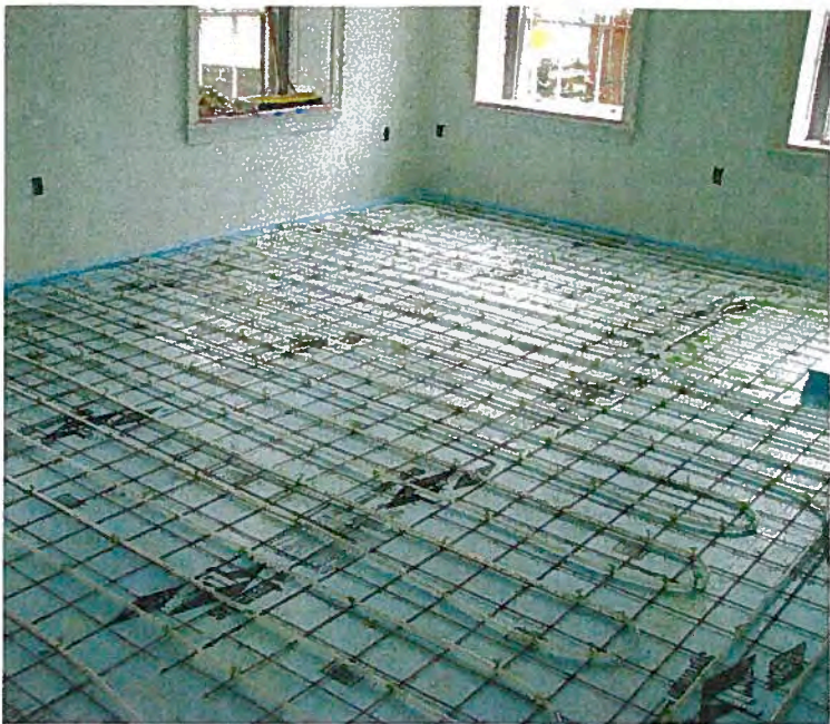
The floor consists of a structural steel deck, 4-inch concrete layer, 2-inch extruded polystyrene and 4-inch capping slab that houses the radiant tubing.
