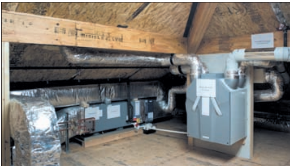
For passive homes that "you could heat with a candle," adequate ventilation is paramount. In this installation two ERVs run continuously, but the air system incorporates an experimental ground loop to temper the incoming fresh air.
