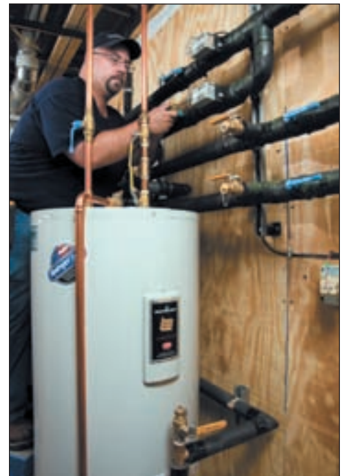
Foley technician, Brian Golden, adjusts a system that incorporates two 50-gallon Bradford White water heaters behind the preheat tank.
